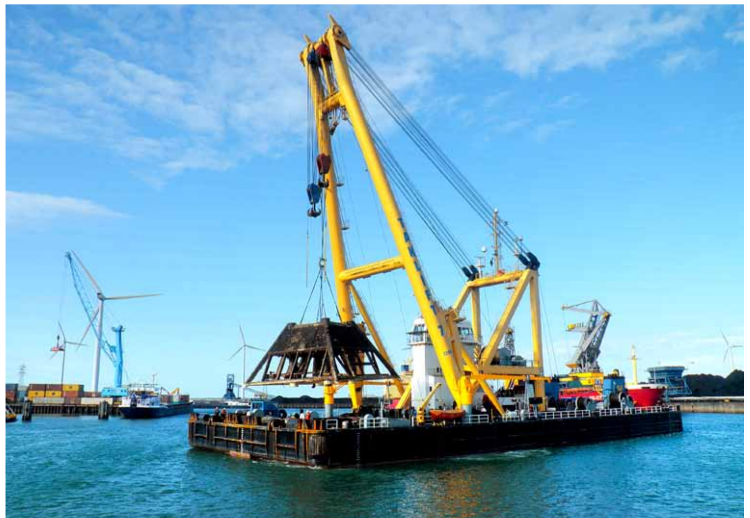
When the structure was lifted, it was brought to Flushing on board 'Taklift 7'.
