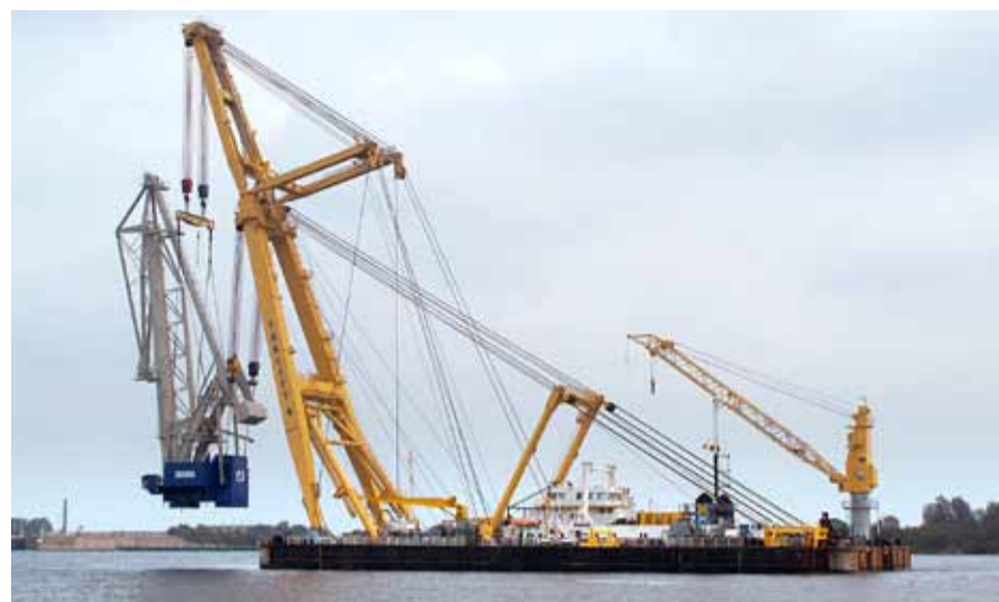
Taklift 4' with one of the two crane topsides in its hooks at Wilhelmshaven.
