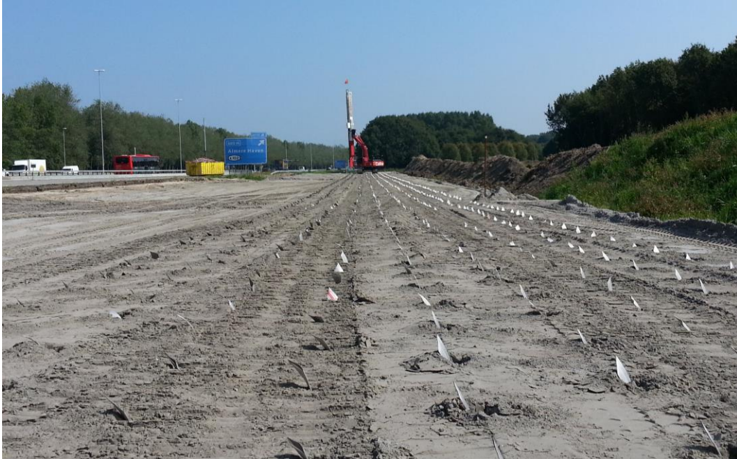
Figure 9. Example of GPS based installation of PVD without the use of pre marking on the ground.
