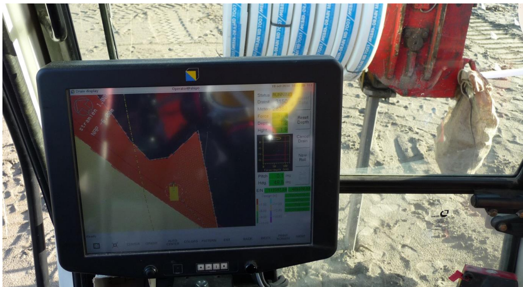
Figure 2. View of the operator screen with on the left the section showing a top view and on the right the real time installation data
